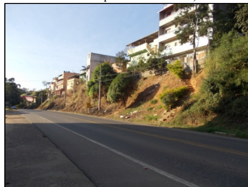
Ponto 28 (Talude com declividade superior a 40%).
